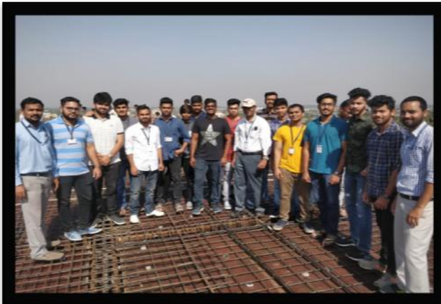
Post Tension Slab Casting, St. John college of Humanities and science, palghar, B.E CIVIL 23 rd March 2019
